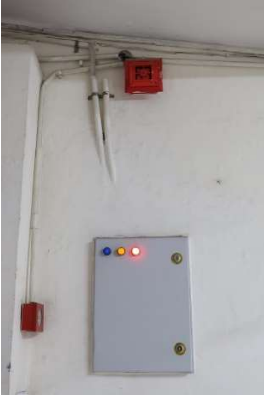
Proper Electricity and Lightning Provision
