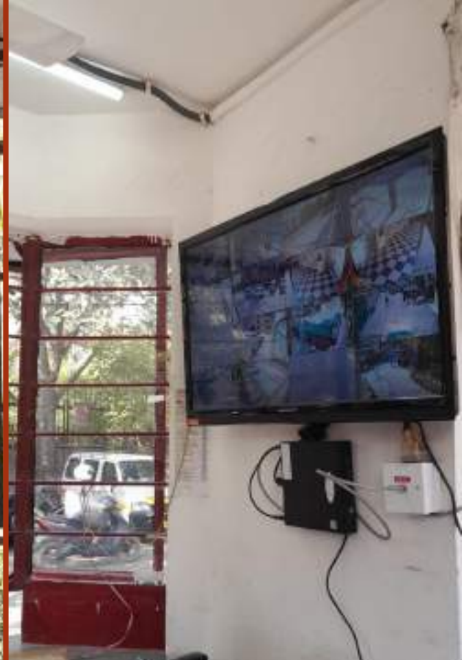
CCTV display in guard room, gate no. 1 at sector 14 - Completed
