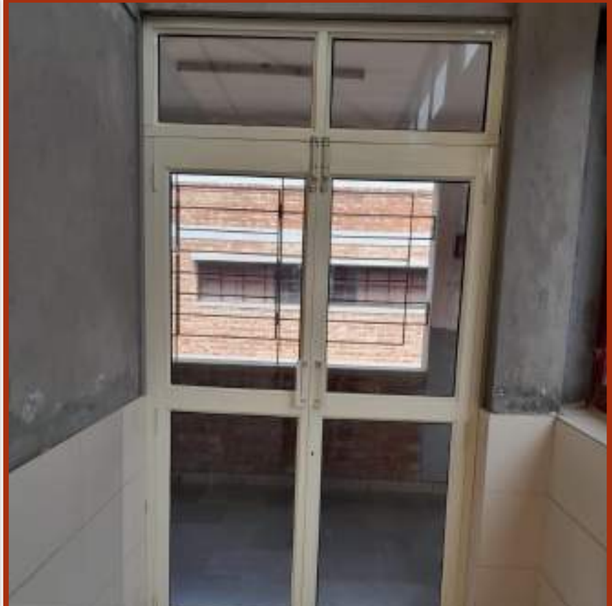
Doors in area under tensile roof, block-II, Top floor at sector 14 - Completed
