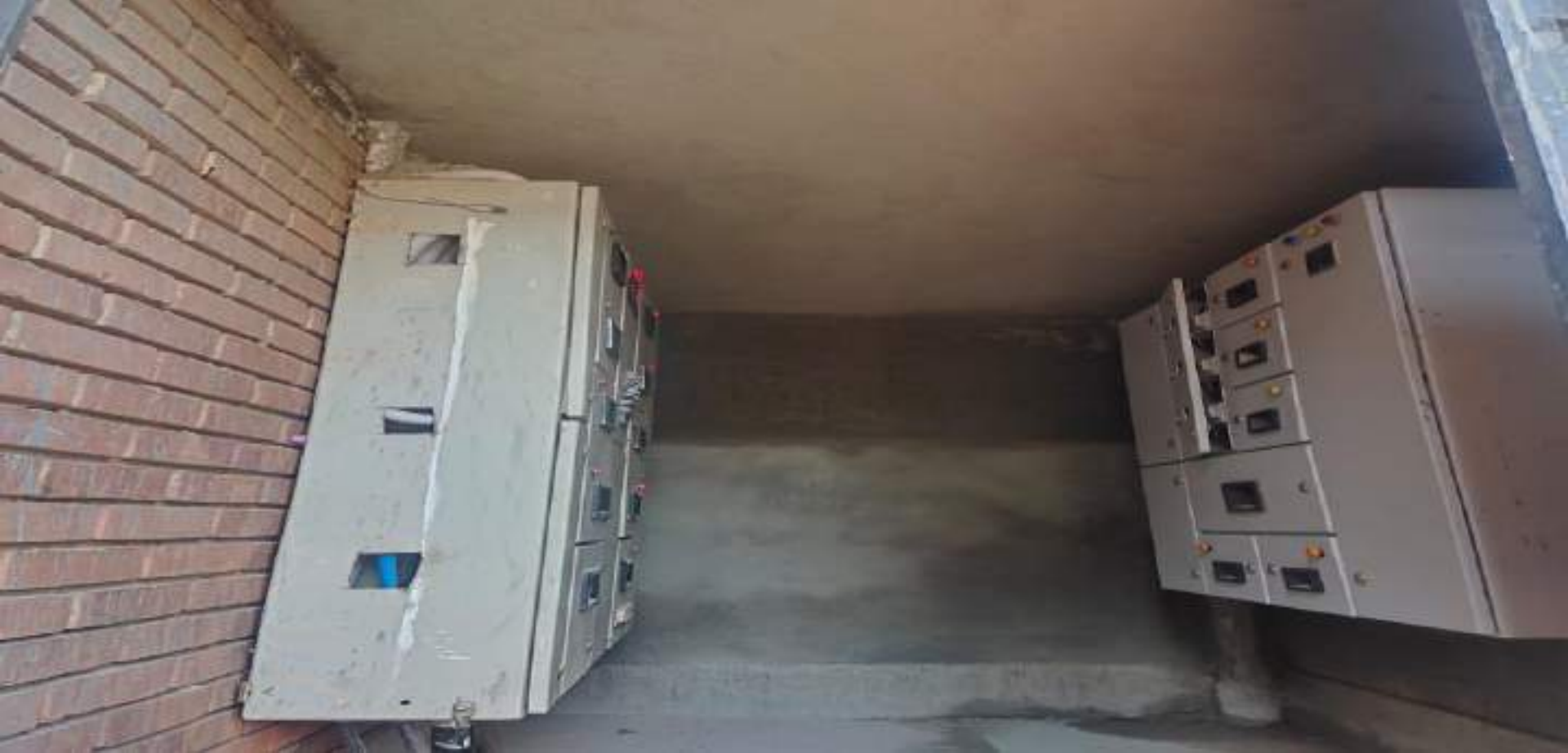
Shifting of Electric Panel Room from Preprimary area, Block I, ground floor – work completed.
