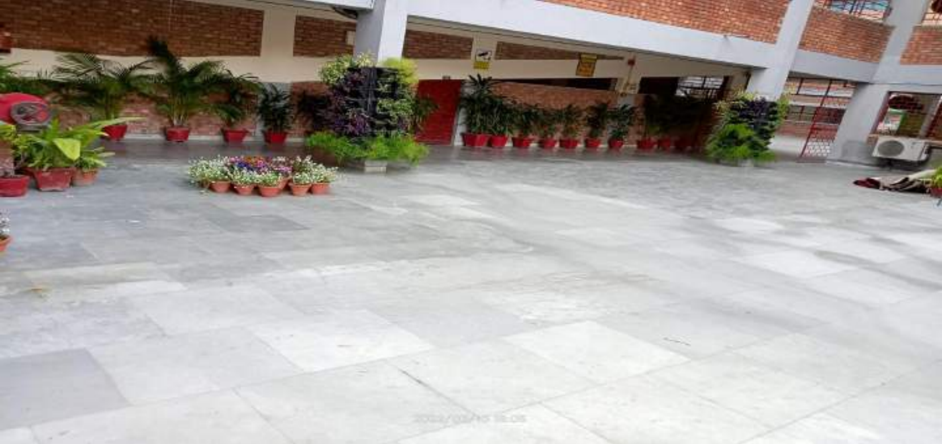
Civil work RCC Slab on open sky shaft near office side, ground floor Block II at sector 14-work completed
