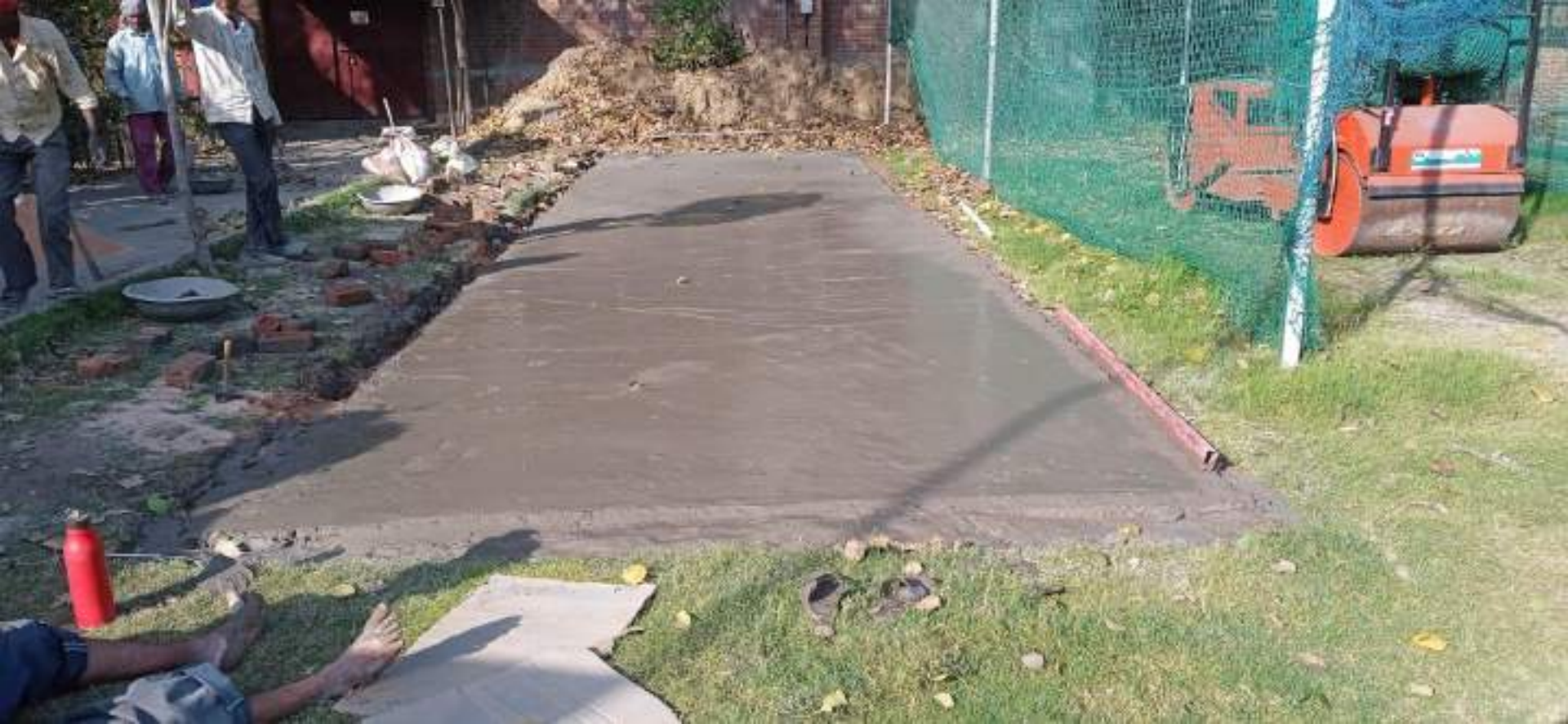
Relocation of Cricket Pitch in playground near Gate no. 3- Work in Progress
