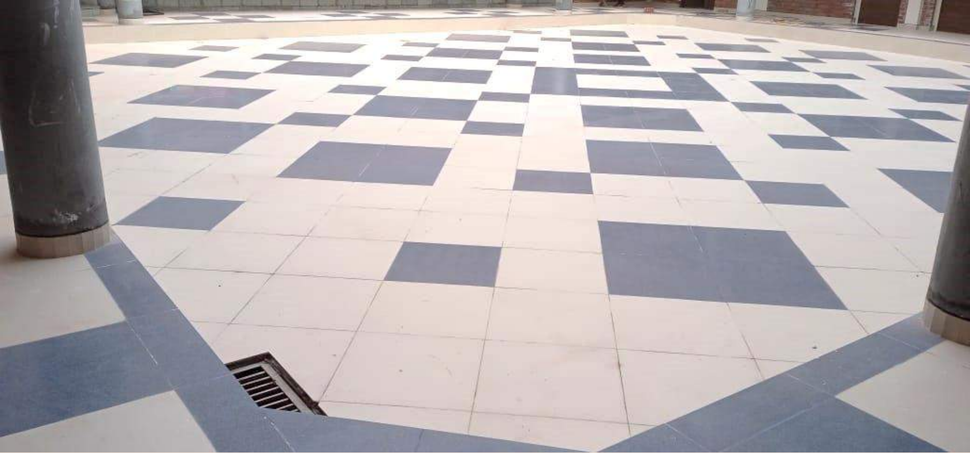
Upgradation of open Courtyard in Block I, Ground floor at sector 14- Work Completed.
