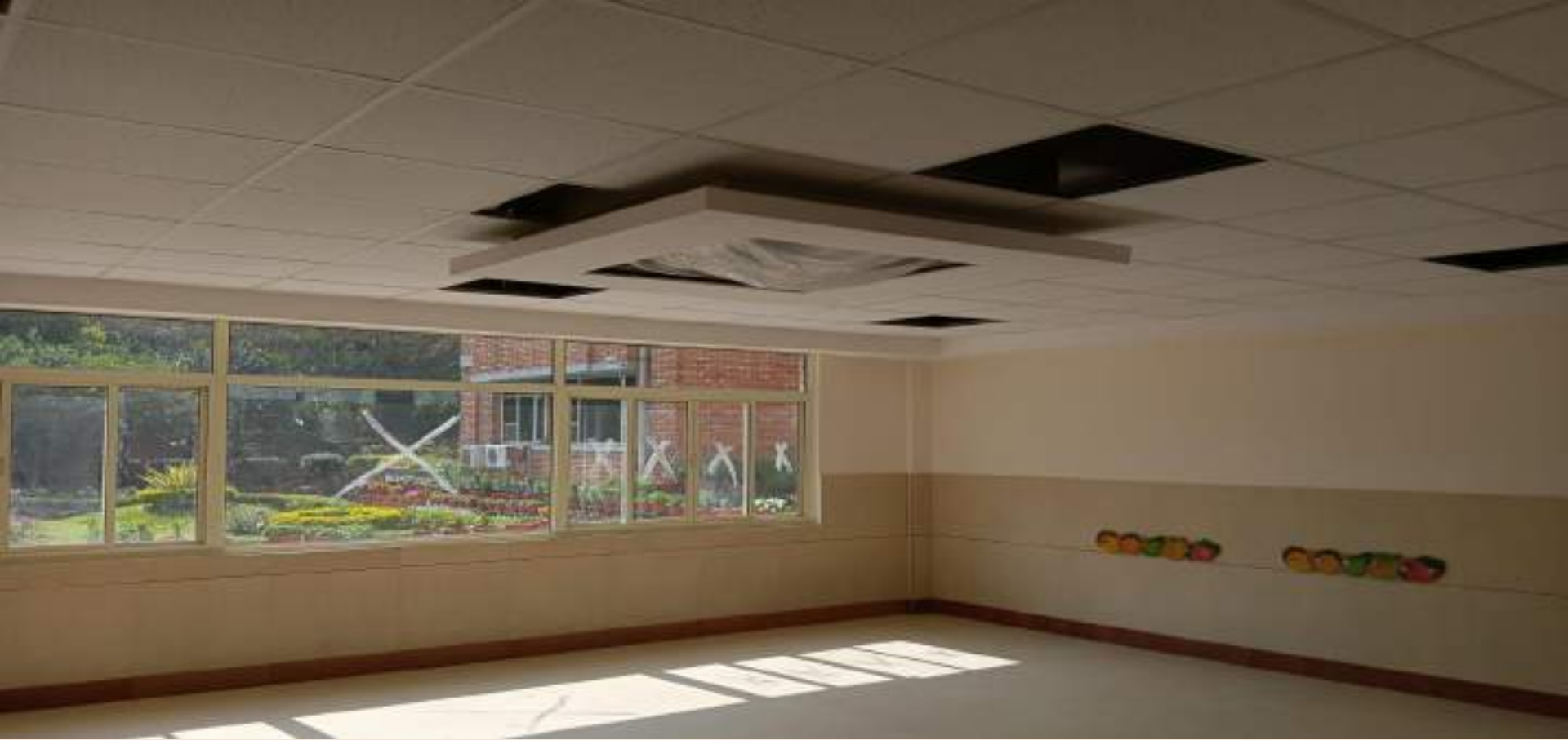
Upgradation of six classrooms in Block I, Ground floor : False Ceiling, Double Door, Windows with Aluminum frame, Cassette AC at sector 14- Work Completed
