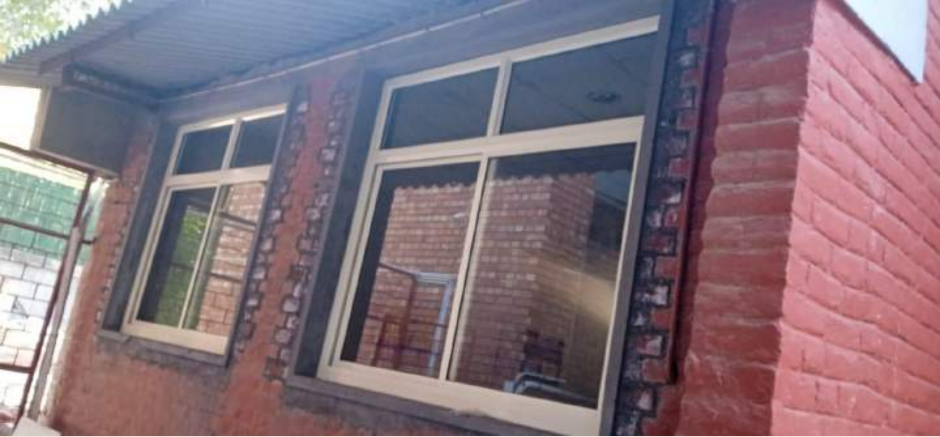
Upgradation of four classrooms in Temporary Block at sector 14- Work in Progress
